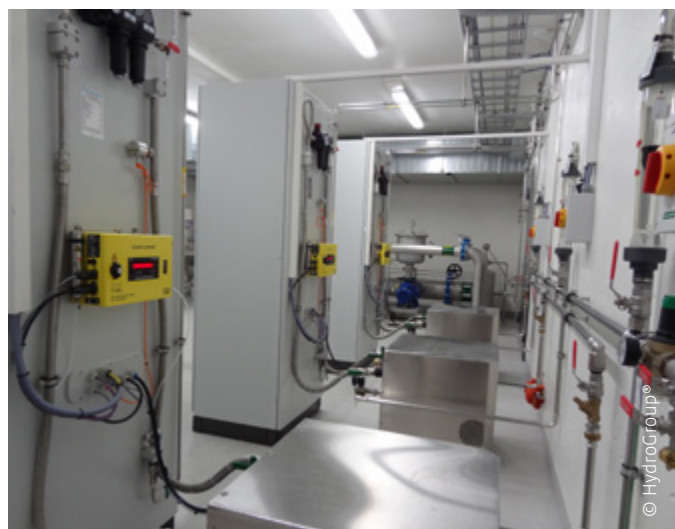
Figure 3: Plasma ozone generators with cooling systems
